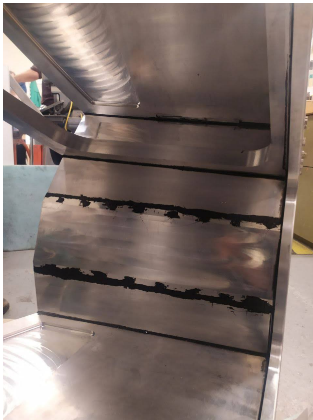
Figure 14: The sealant on the bottom panels before scraping, for comparison.
