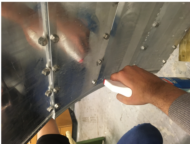
Figure 6: The soapy water test is done by spraying soapy water over the seams.
