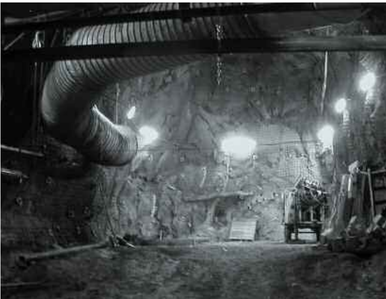
Excavation for the new SNOLab facility near Sudbury, Ontario, nearly 2 km underground.
