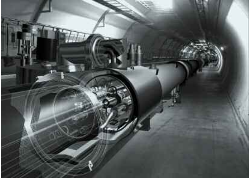
A mock-up of the LHC tunnel at CERN showing the two beam pipes in which the 7 TeV proton beams will travel around the 27-km ring.
