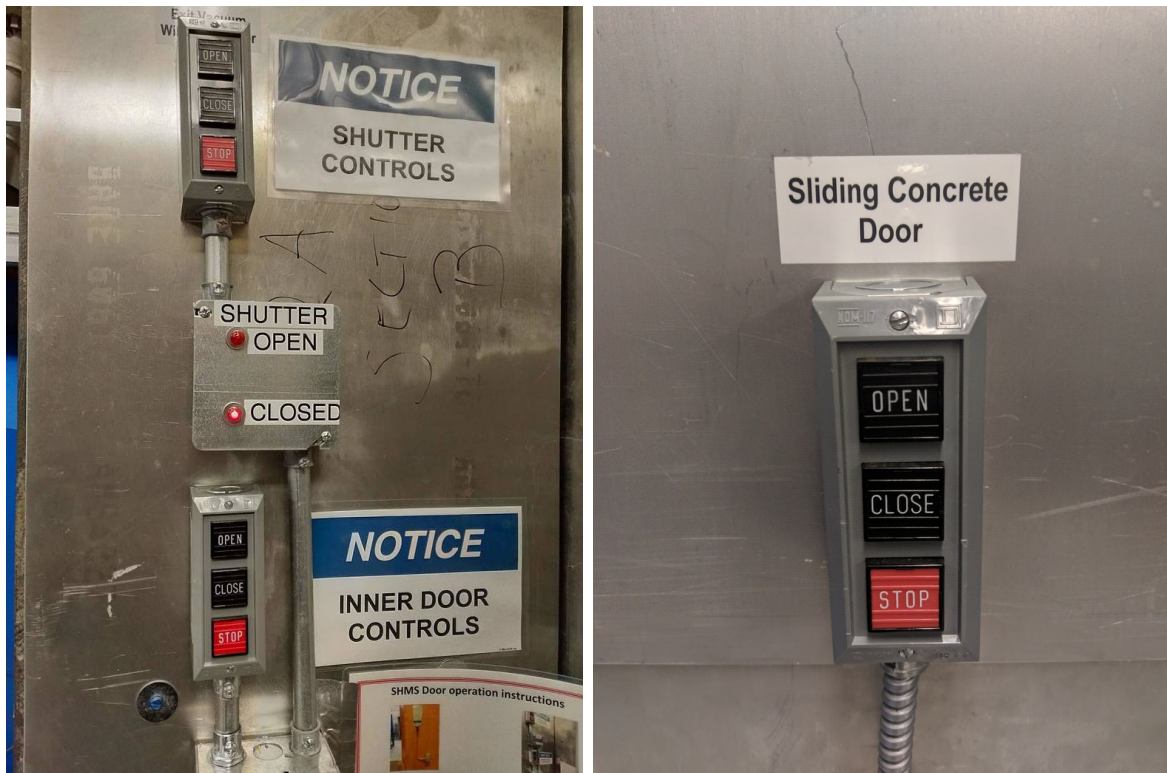
Figure 5.13: SHMS barn door controls. The left picture shows the controls located in electronics hut. The bottom buttons control the barn door. The top buttons control the SHMS vacuum extension shutter. Below the shutter controls are lights indicating if the shutter is opened or closed. The right picture shows the barn door controls located inside the detector hut.
