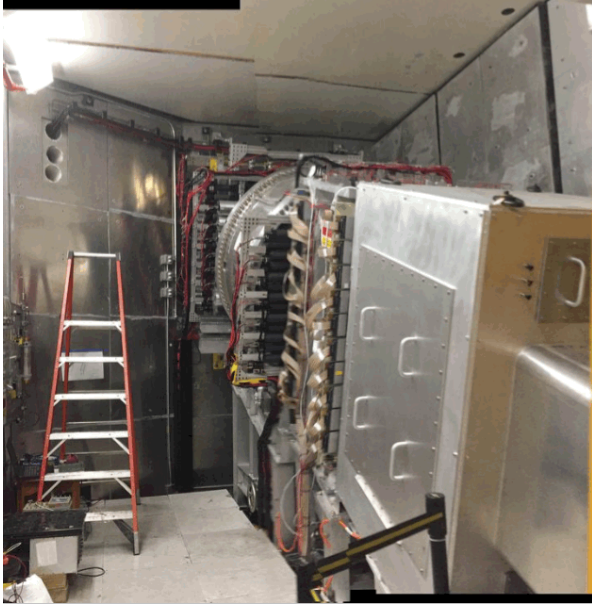
Figure 62: Photo of the SHMS Detectors in the Shield House
