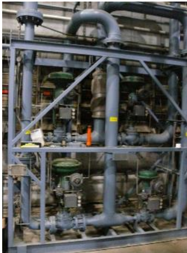
Figure 11.9: Gas management system with control valves.
