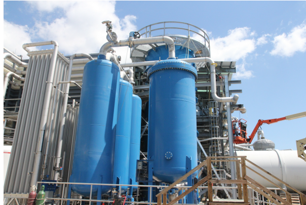
Figure 11.8: Oil removal system.
